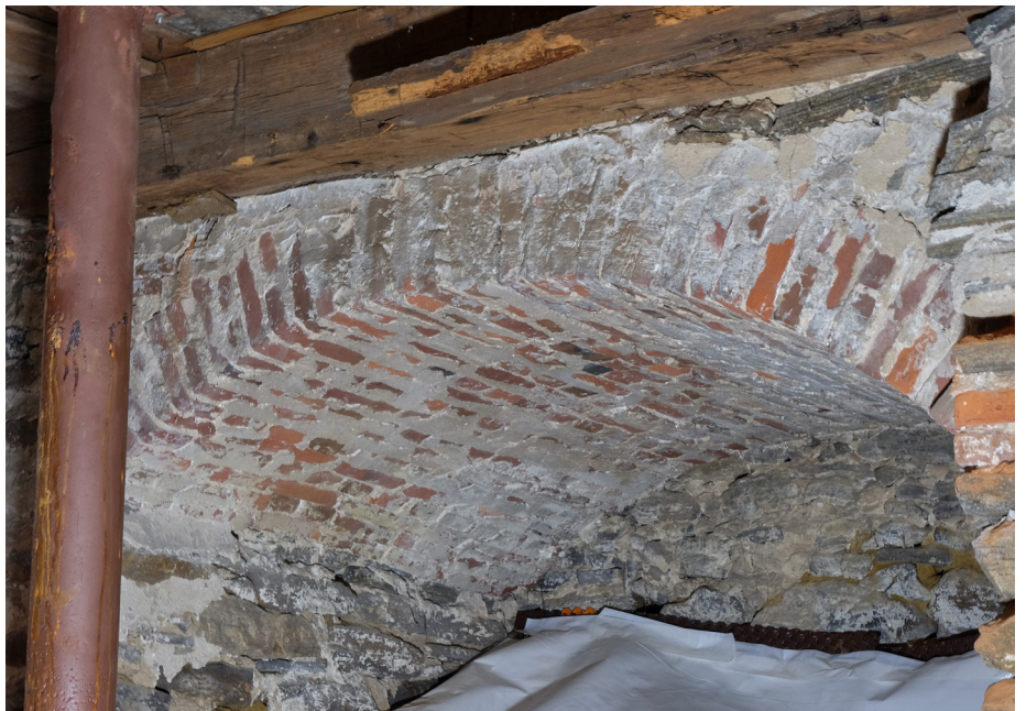
Photo 9. Chimney support under the front fireplace as seen in the basement, 2025 (C. Cielo photograph).
