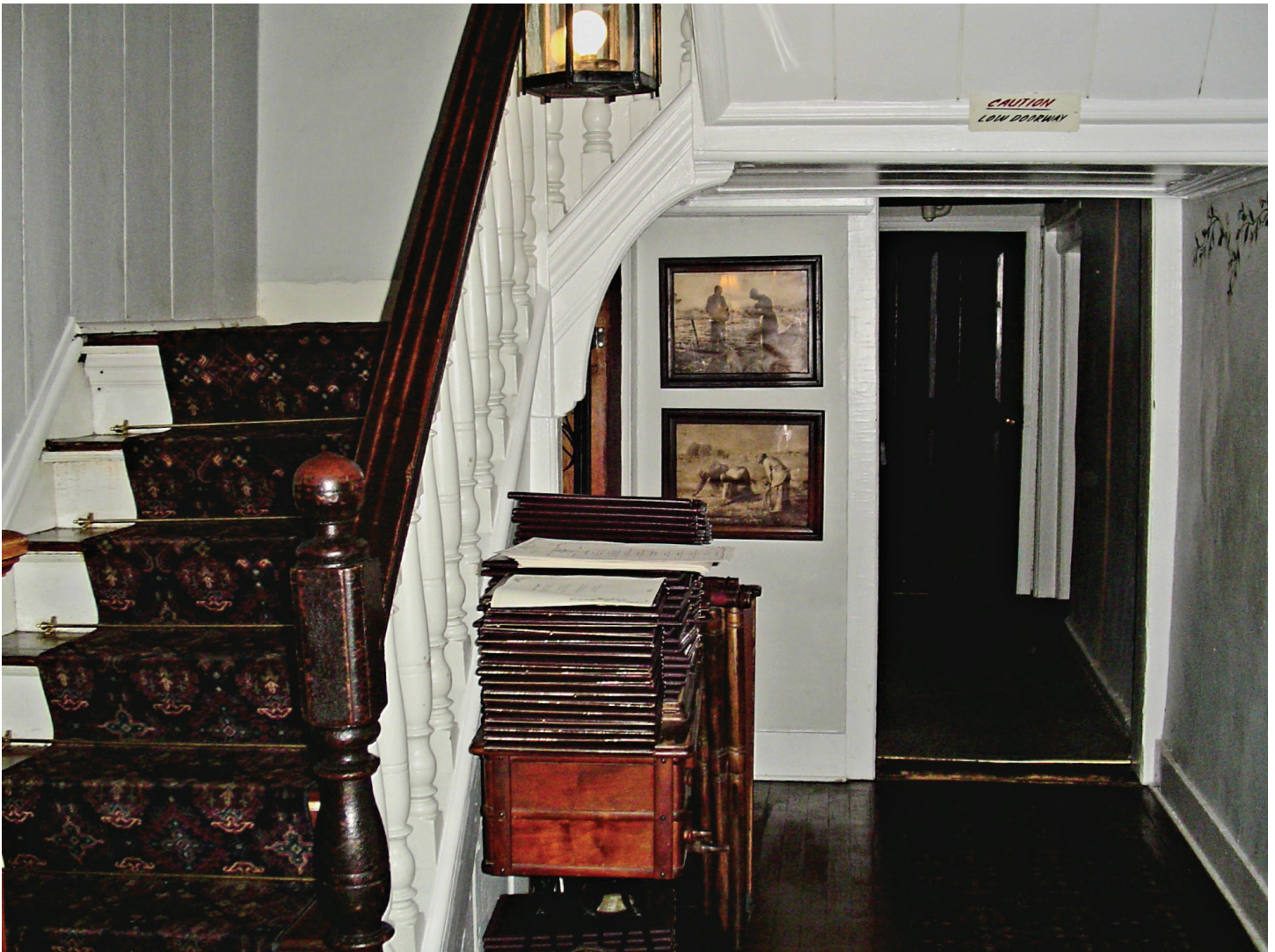
Figure 4. Main staircase in the Glen-Sanders mansion, Scotia, Schenectady County (Author photo, June 2004). The gouge is seen just to the right of the ball finial of the newel post.
